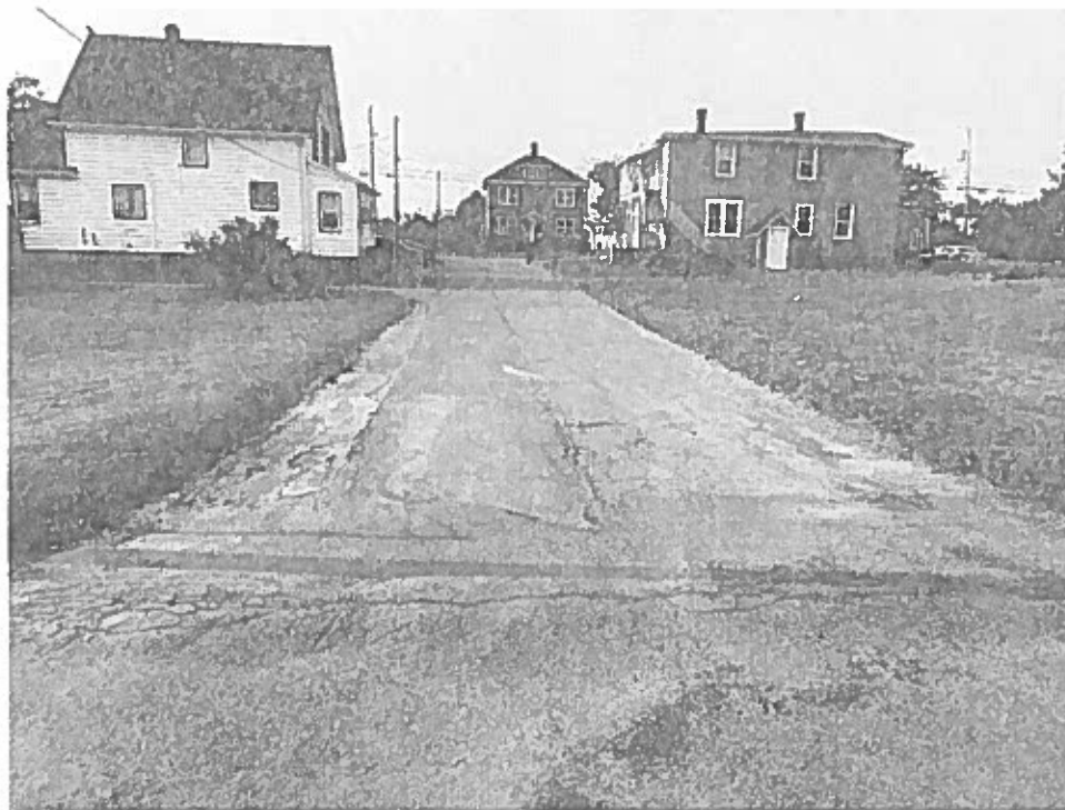
Figure 6: Church St - Insufficient storm pipe cover, cross slope, and drainage - Recommend further investigation.
