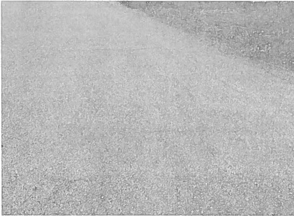
Figure 1: Light cracking and light ravelling
