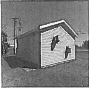
No fire extinguisher
